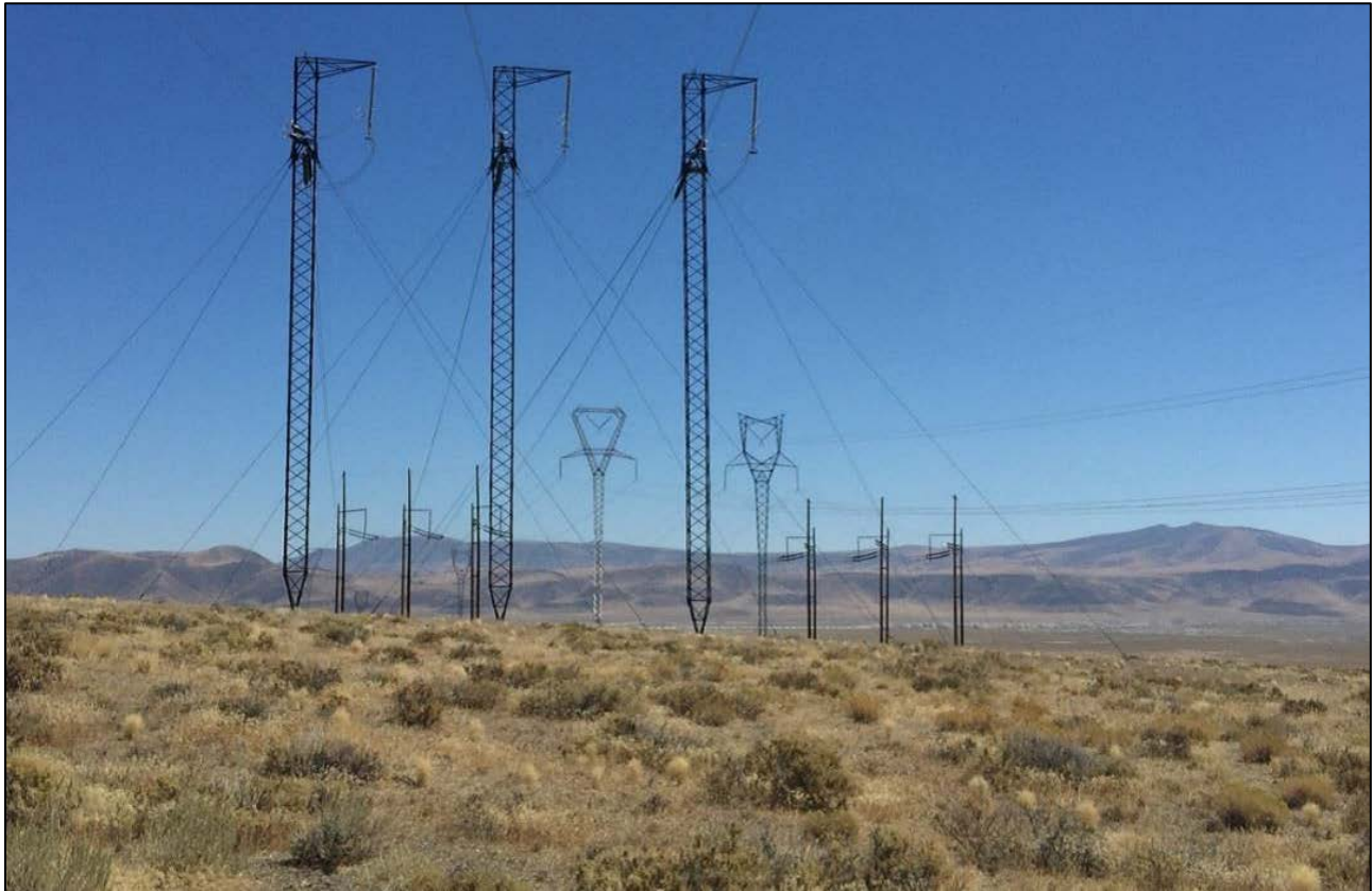
Existing high-voltage transmission lines near proposed substation location (Photo courtesy of Dodge Flat Solar LLC)
